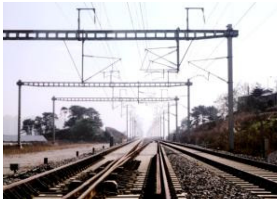
KTX infrastructure, Republic of Korea
